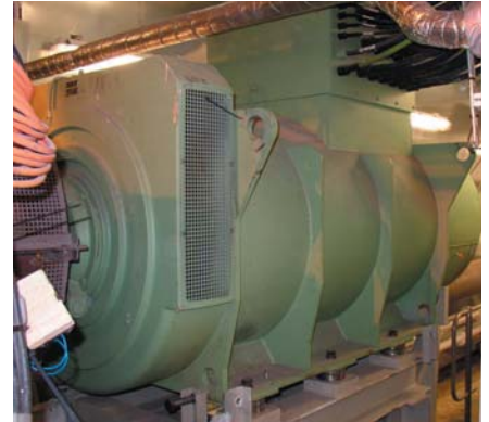
PTO shaft generator
