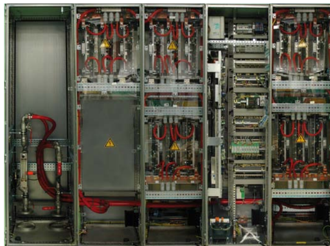
Inner view of the converter at the terminal
