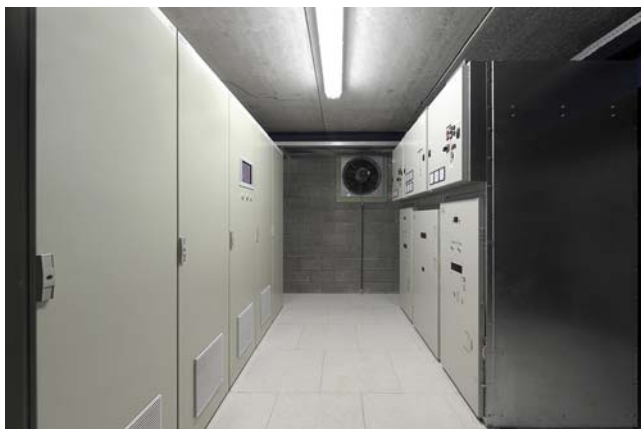
Frequency Converter and switchboard at terminal
