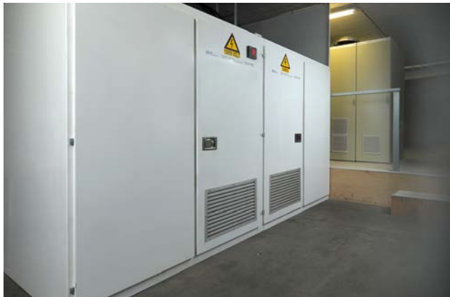
Transformer at terminal
